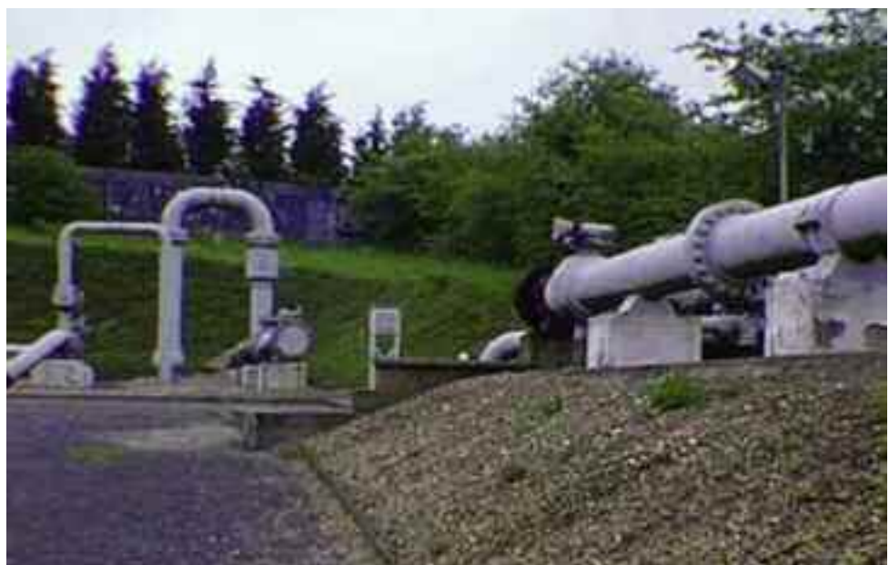
Figure 3 Surface pipelines within an oil fuel depot
