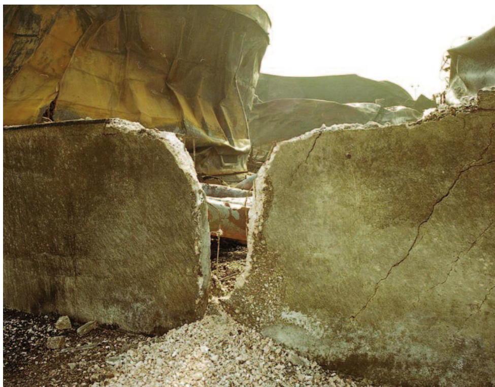
Figure 8 Failed bunds on the Buncefield site photographed after the fires were all out
