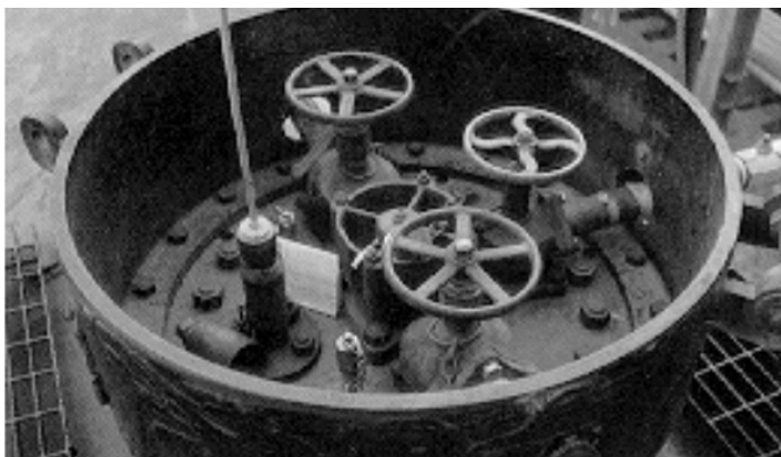
Close-up of typical LPG tank car dome, showing liquid and vapor connections and magnetic level gauge.
