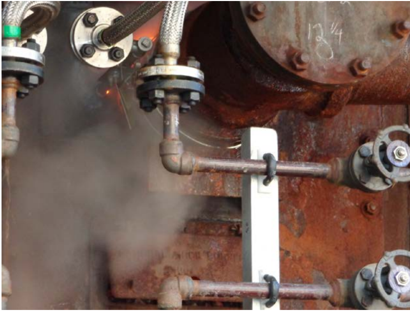
FIGURE 7. Burner on furnace (Source: CSB).
