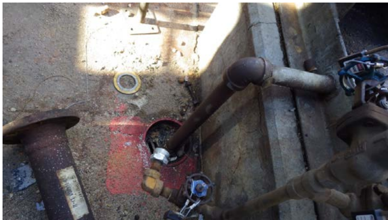
FIGURE 8. Typical pump drain to OWS (Source: CSB).
